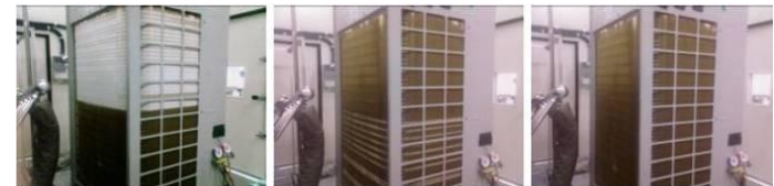
Lower defrost Upper defrost Lower defrost
