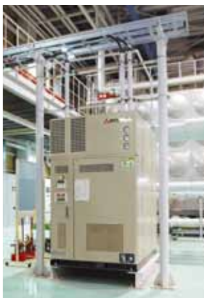
Heat recovery heat pump water heater
