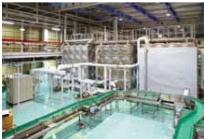
Heat recovery heat pump water heater and hot water tanks. From the left: high-, medium-, and low temperature water
