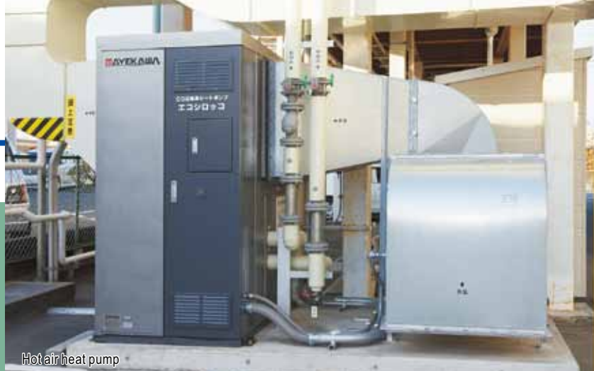
Hot air heat pump
